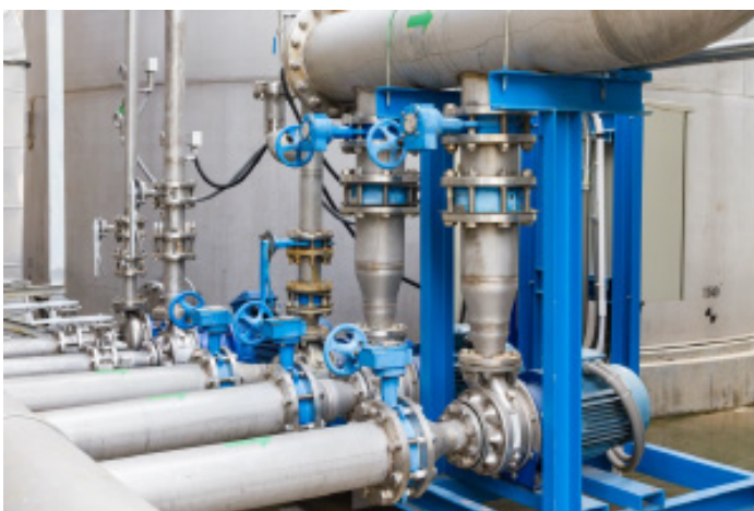
Figure 1: Upon detecting an abnormality in operation, monitoring relays switch equipment off until maintenance can be supplied.
